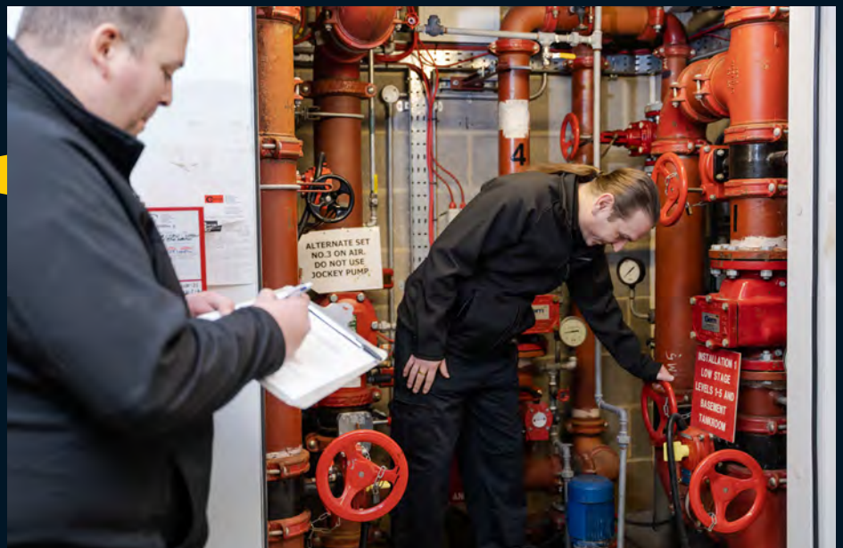
Introducing the team at One London Wall. From top left to right: Ian Pease, Site Manager; Gavin Watt, Handyman; David Chapman, Electrical Technician and Matthew Penny, Mechanical Technician
